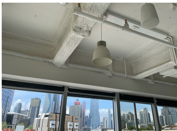
Fig. 1 Structural steel was required to strengthen the concrete slab. Access to the floor below the scanner needed to be negotiated with the tenant. Despite the increased cost, patient, and staff amenity of a department with access to natural light, not to mention views is considered to be an advantage of locating imaging departments above ground rather than their traditional basement positioning
